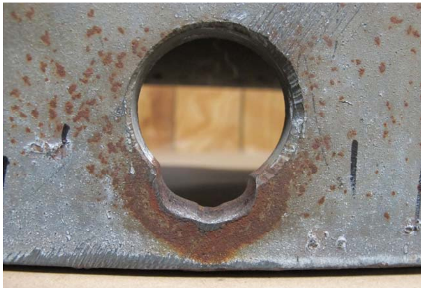
Figure 7: The as-received condition of the eye of Sample 1-1. The material appears to have yielded though the excess material seems to have been chipped off of the front of the eye. The wide area of wear suggests that the Y-bolt may have been rocking and swaying over an extended period of time in the field.
